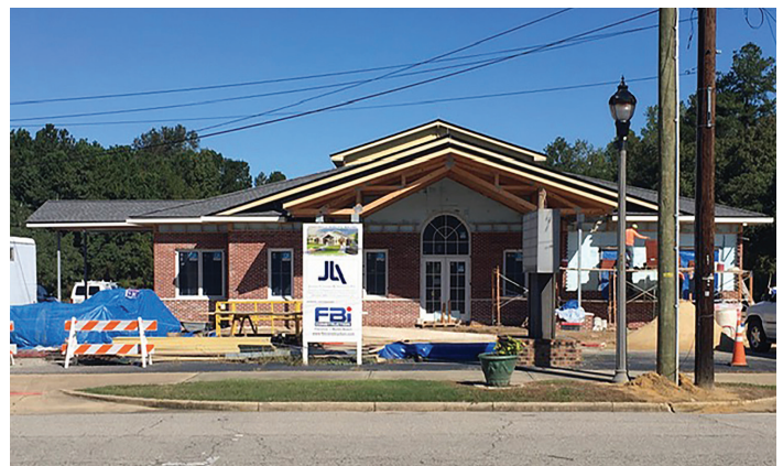
Johnsonville has built a new city hall where a vacant grocery store had once stood. Photo: City of Johnsonville.
