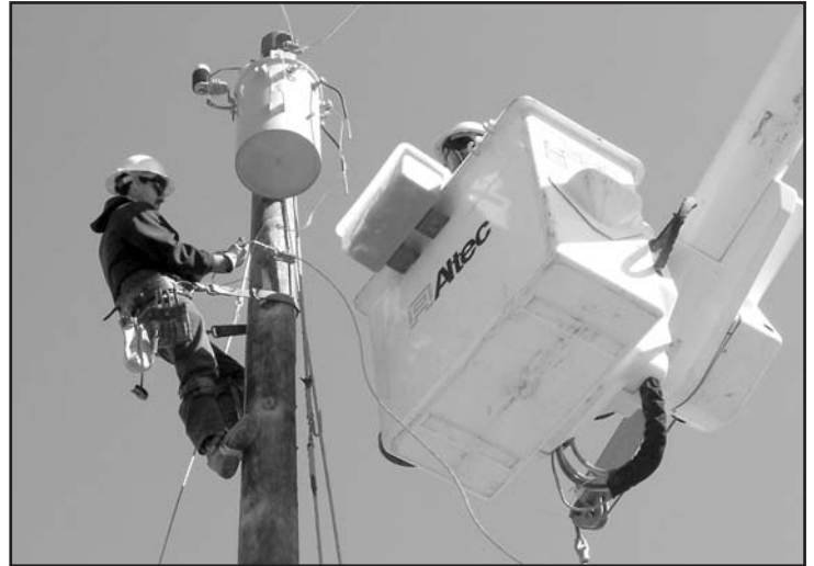
A lineman from Easley Combined Utilities works to restore power after the December 15 ice storm.
