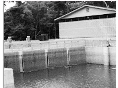
To help alleviate flooding problems, stormwater is pumped into a 13-acre lake through four 48-inch pipes. The lake is surrounded by a community park.
