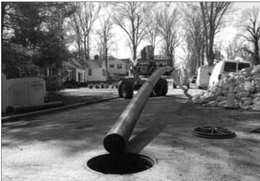
The City of York replaced some of the oldest water and sewer infrastructure in the City by using pipe bursting, a trenchless method of sewer infrastructure replacement.
