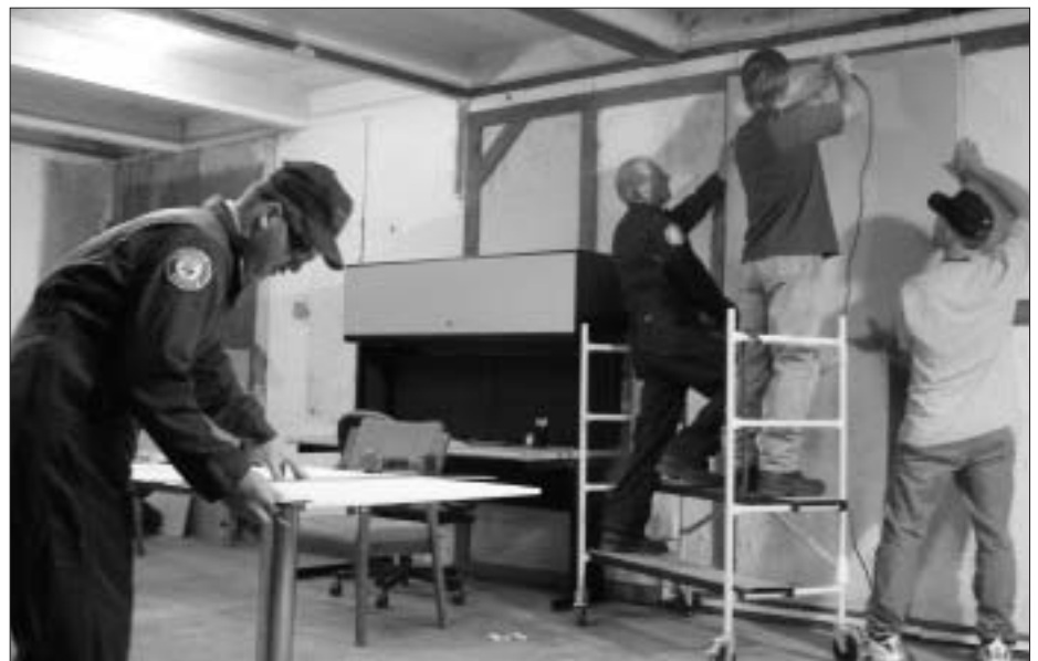
Twenty-five volunteers and 12 paid firefighters spent more than 2,500 hours working to renovate the City of Woodruff's abandoned National Guard Armory into a fire station.
