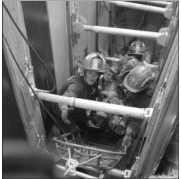
Using a 28-foot trailer, Lancaster firefighters can transport its special excavation equipment to assist in trench construction and rescues.
