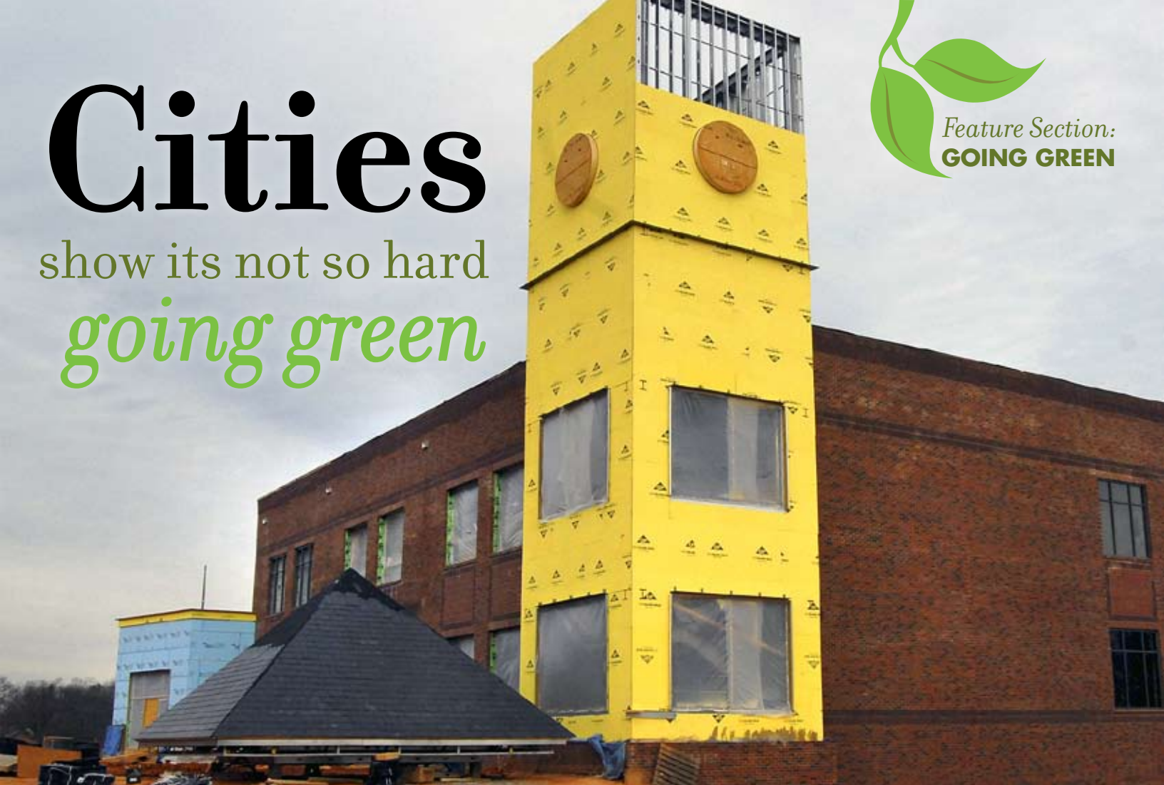
The Greer City Hall, currently under construction, is situated to give stairwells and offices full advantage of natural light.
