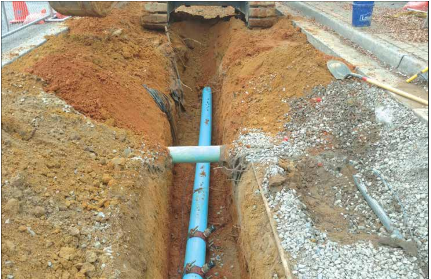
The City of Aiken's Newberry Street Phase 1A Project included improvements to stormwater infrastructure. Photo: City of Aiken.
